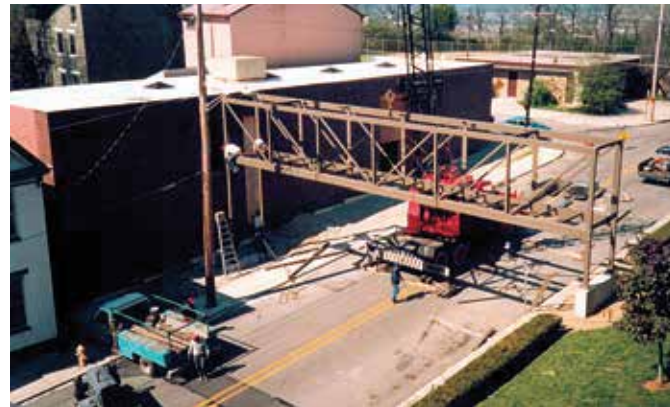
[below] Construction of the skywalk connecting the new library to main campus.
