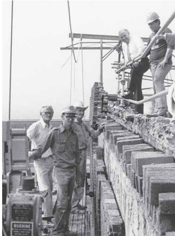
[left] David Rodgers, Ricky Moody, Carl Antrim, President Miller and Wayne Via. Reconstruction of the parapet wall of the Revivalist Memorial Building was the first step in major renovation of that building.
